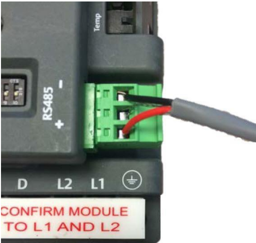
Figure 50 CoreSense Diagnostics Modbus Connection
